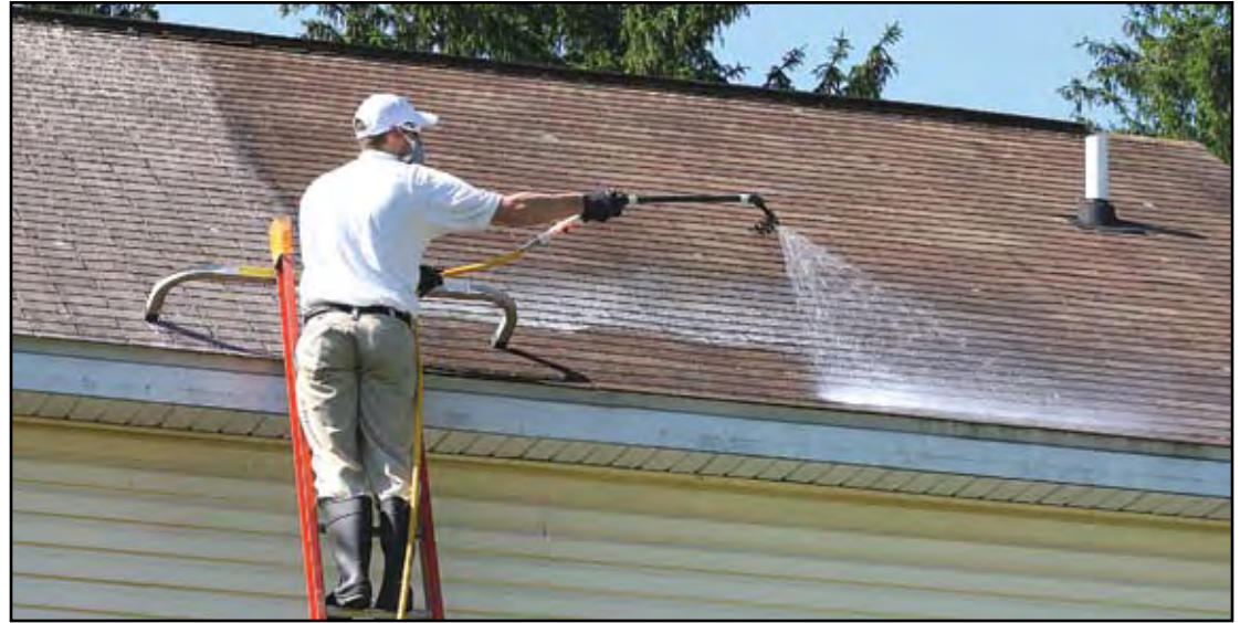
Dan Cronauer, owner of Apex Roof Cleaning, sprays the soft wash solution on a roof top in Luzerne County.
